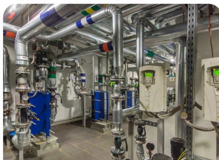
MECHANICAL Booster sets, pumps & pressurisation
