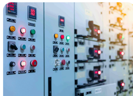
CONTROLS MCC panels, BMS & vessels
